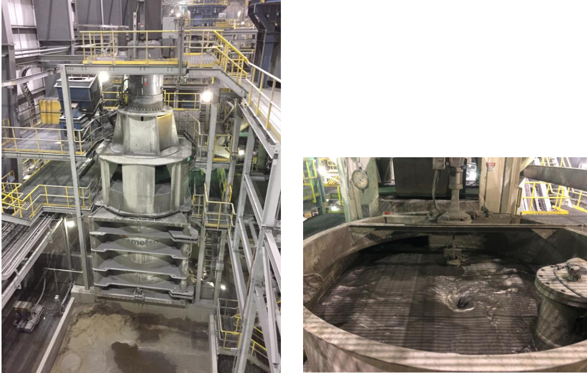
Figure 7 – Vertimill and Separating Tank
